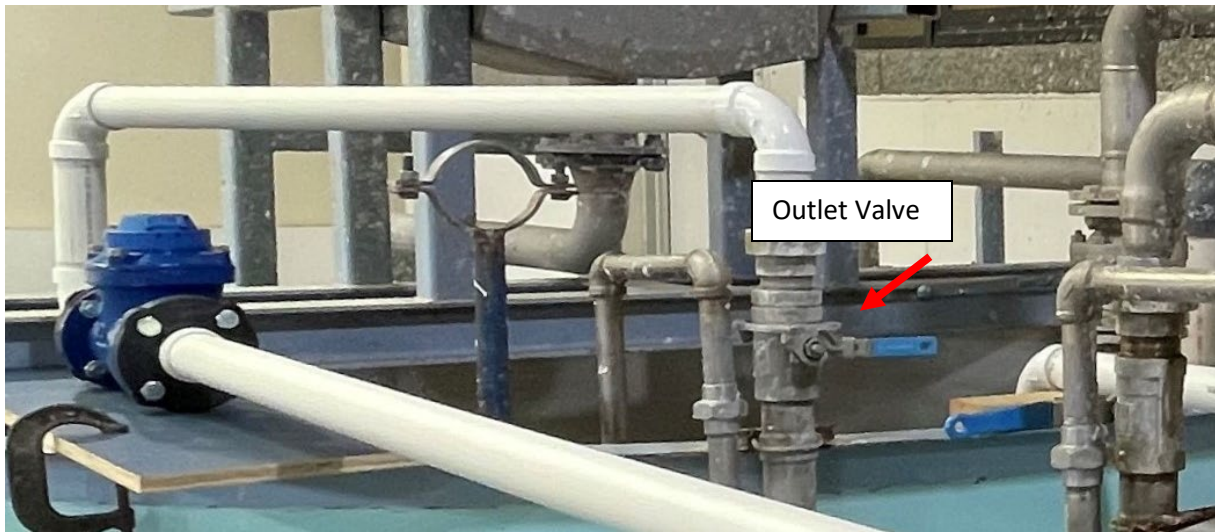
Figure 2. House water inlet valve and test flow loop
